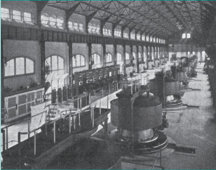
figure 9. Power House No. 1 contained 10 vertical shaft turbines, each driving an identical 5,000-hp alternator. The end user was required to convert the power to fit their needs. (Source: George W. Davenport, Niagara Falls Electrical Handbook , AIEE, 1904; in the public domain.)
