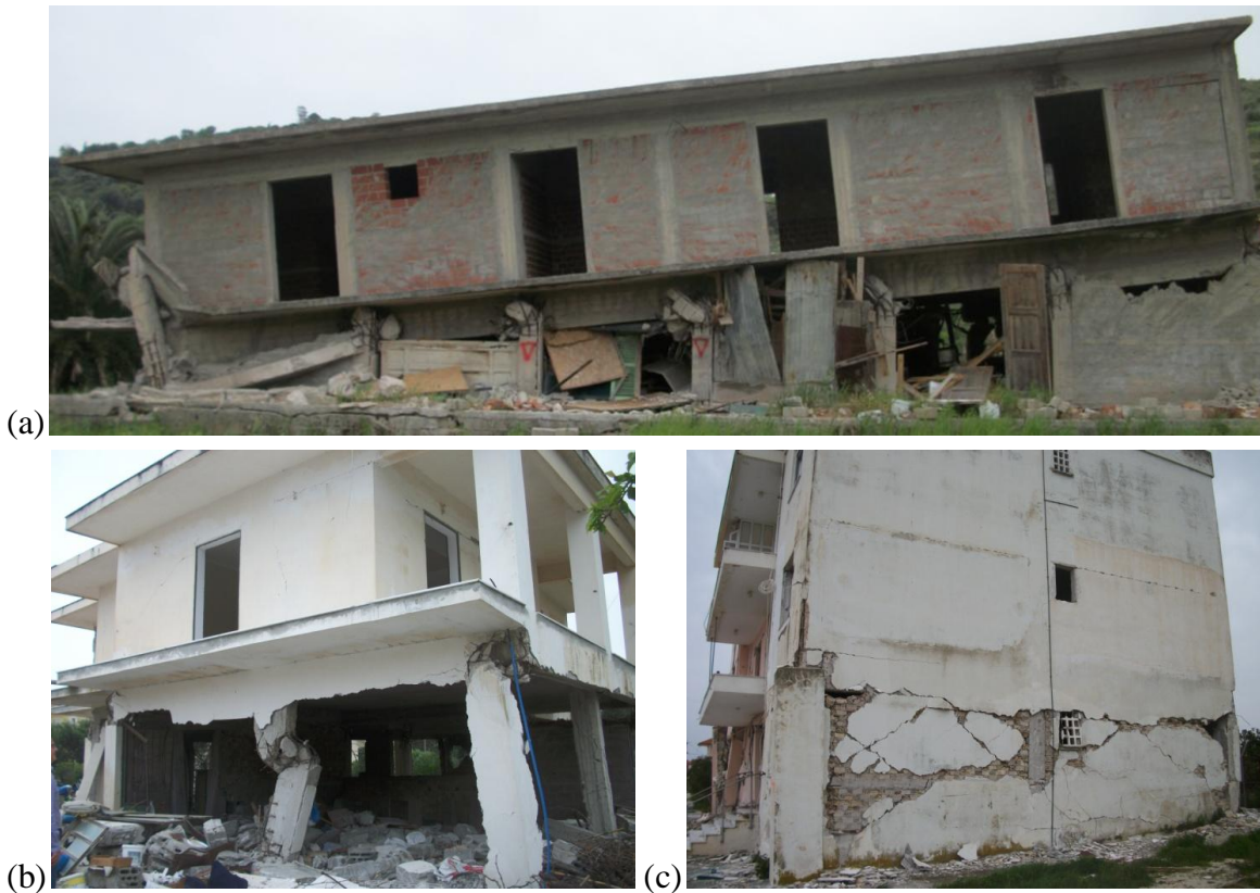
Fig. 2.14 Typical concentration of failures or damage in ground storey with role and damage to infills shown in (c).
