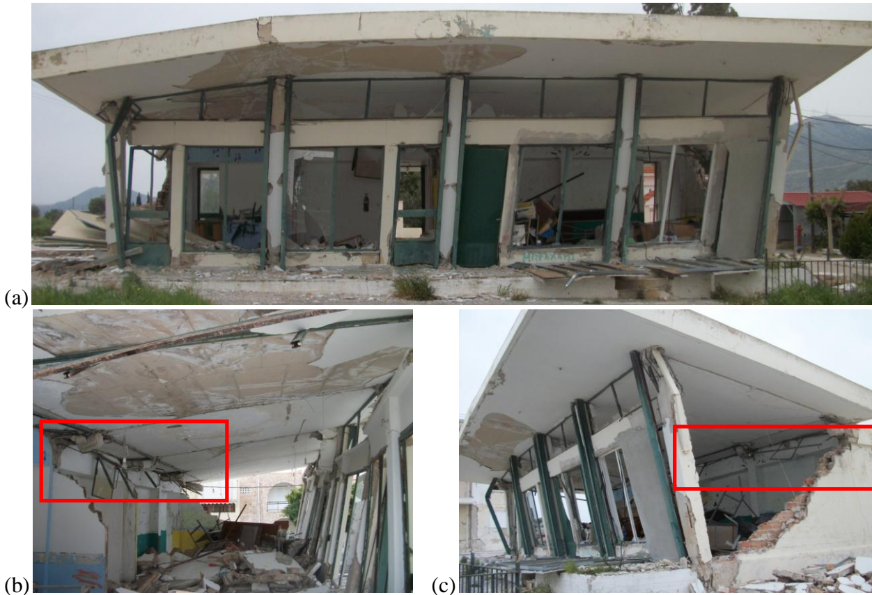
Fig. 2.17 Shear failure of short columns on stiff side (inside red rectangle) causes collapse of flexible side as well.
