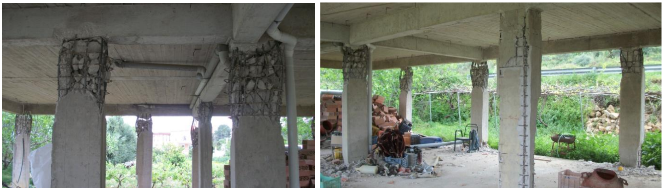
Fig. 2.20 Despite complete failure of columns across the ground storey, their residual axial load capacity still supports gravity loads.
