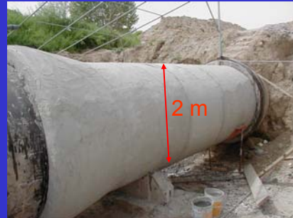
Confinement of leaking water-pipe (Thessaloniki, Fyfe Europe s.a.)
