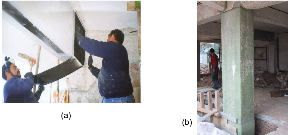
Fig. 5.3 Shear strengthening (a) of beam end with CFRP, (b) of column with GFRP.
