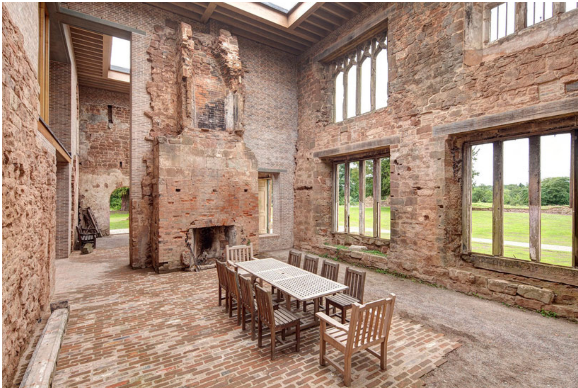
main hall exemplifying moments of the new intervention and the old construction
