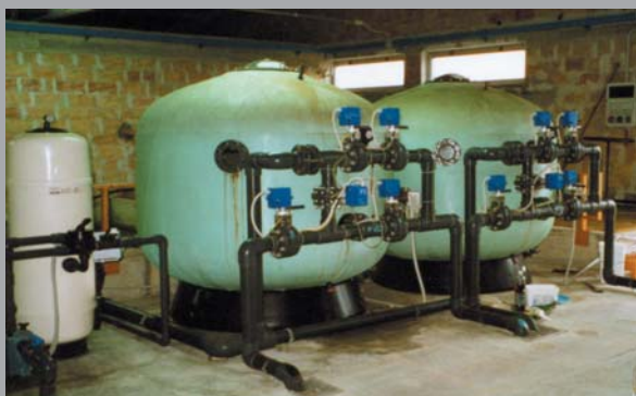
Fig. 24.01 Mechanical sand filter for the water inlet (photo STM Aquatrade)
