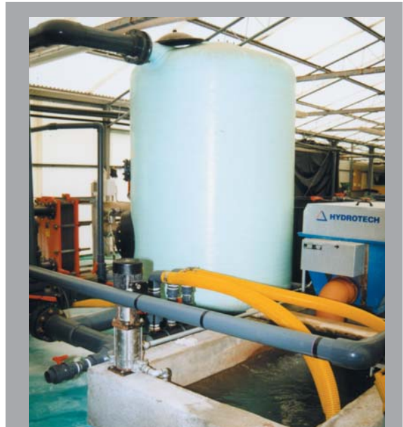
Fig.68.01 Well cleaned biofiltration unit (photo STM Aquatrade)
