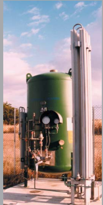
Fig.58.01 Small liquid oxygen reservoir sized for hatchery need (photo STM Aquatrade)
