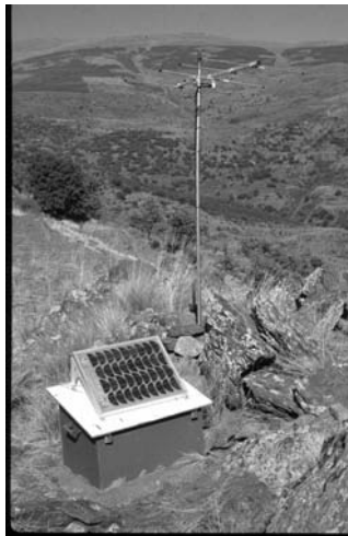
Figure 7.15 A small 12 W mono-crystalline solar panel mounted on top of the case of a temporary seismic station. Both sides of the panel are light sensitive, so the roof of the case is white-painted to reflect the diffuse radiation to the rear side of the panel.
