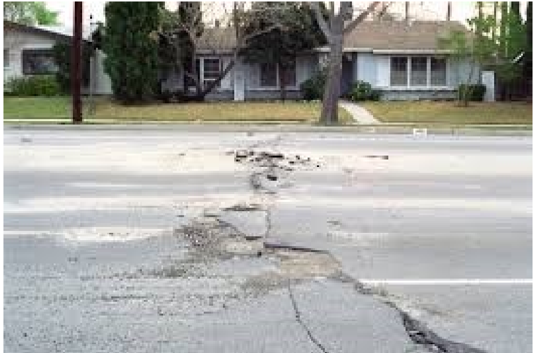
http://en.wikipedia.org/wiki/1994_Northridge_earthquake#/media/File:Street_Damage_After_Northridge_Earthquake.jpg Street damage after the Northridge Earthquake of January 17, 1994.
