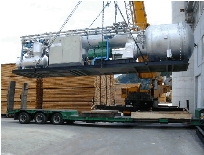
Figure 8 The Admont (Austria) T450-CHP unit during installation on site in 1999 (Source: Turboden)
