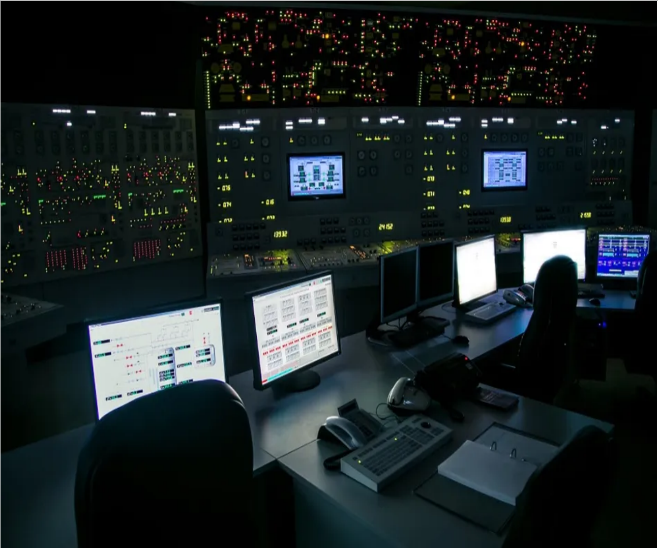
lock control panel of nuclear power plant operates on a backup power supply during an accident simulation
