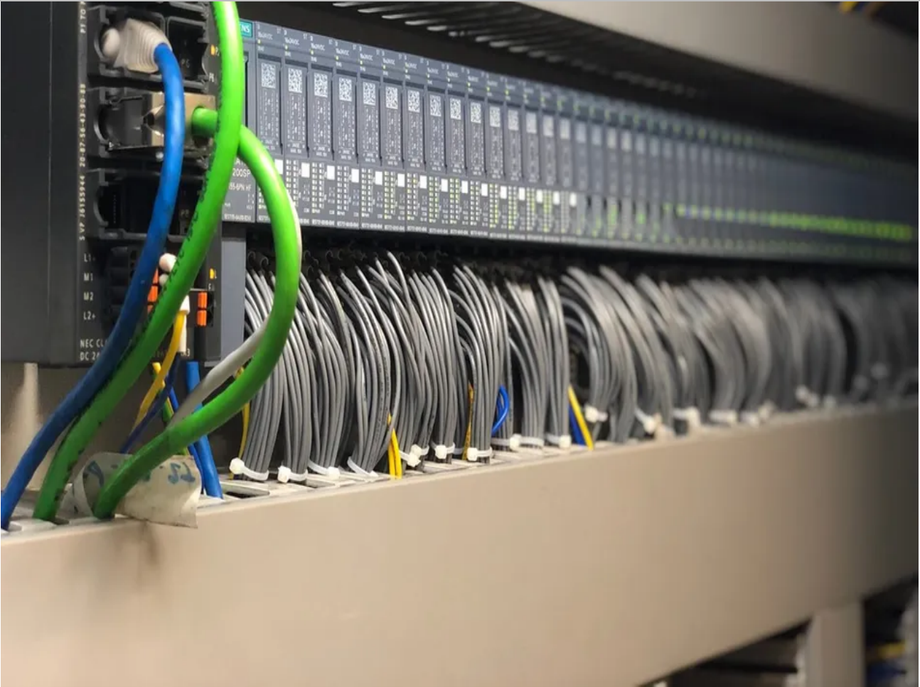
Programmable Logic Controller(PLC) being used in water treatment system control
