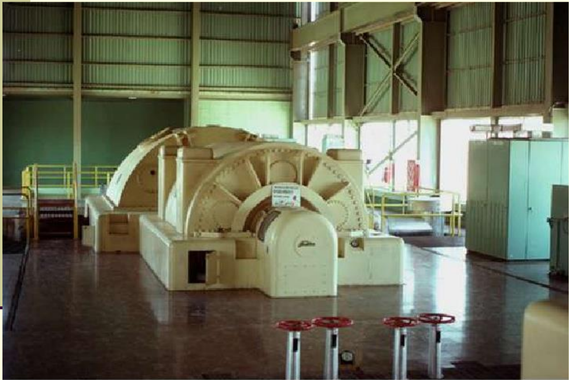
Turbine generator in a geothermal power plant in Cerro Prieto, Mexico.
