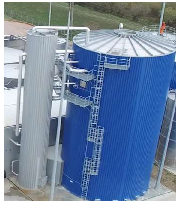
ECSB reactor - AquaThane LTD
