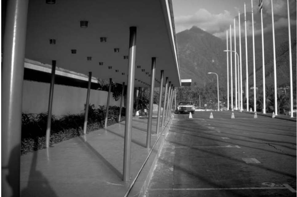
Figure 1.1.1 This pergola at the Macuto-Sheraton Hotel near Caracas, Venezuela, was damaged by earthquake on July 29, 1967. The Magnitude 6.5 event, which was centered about 24 km from the hotel, overstrained the steel pipe columns, resulting in a permanent roof displacement of 22.86 cm. (From the Steinbrugge Collection, National Information Service for Earthquake Engineering, University of California, Berkeley.)
