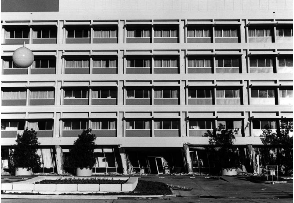
Figure 20.3.4 Large deformations in the first aboveground story of the Olive View Hospital building due to the San Fernando earthquake of February 9, 1971. (Courtesy of K. V. Steinbrugge Collection, Earthquake Engineering Research Center, University of California at Berkeley.)
