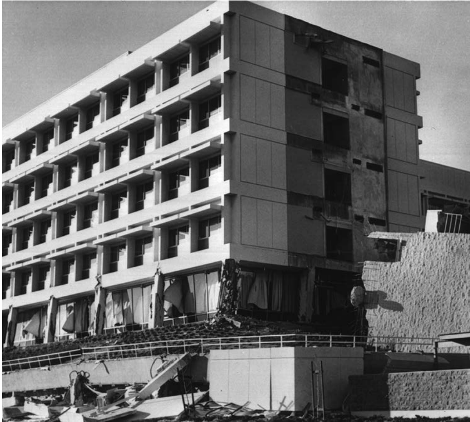
Figure 20.3.3 Olive View Hospital building. The shear walls in the upper four stories did not extend to the lower two stories. (From K. V. Steinbrugge Collection, courtesy of the Earthquake Engineering Research Center, University of California at Berkeley.)
