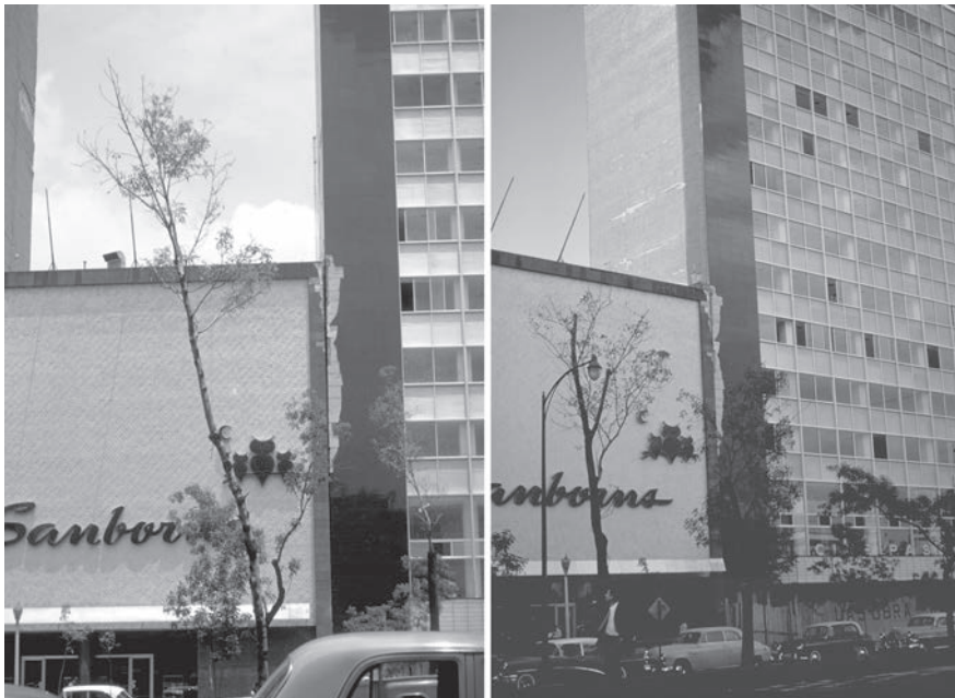
Figure 6.3.1 Two images of pounding damage to the Sanborns Building (shorter) and 33 Reforma Avenue Building (taller), Mexico City due to Mexico earthquake of July 28, 1957. (From the Steinbrugge Collection, National Information Service for Earthquake Engineering, University of California, Berkeley.)
