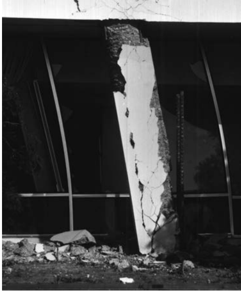
Figure 20.3.6 Large permanent deformation of a spirally reinforced column of the Olive View Hospital building. (From K. V. Steinbrugge Collection, courtesy of the Earthquake Engineering Research Center, University of California at Berkeley.)
