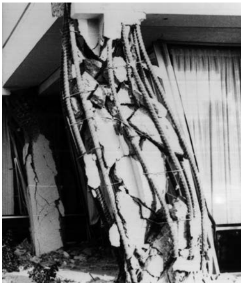
Figure 20.3.5 Brittle failure of a tied corner column of the Olive View Hospital building. (From K. V. Steinbrugge Collection, courtesy of the Earthquake Engineering Research Center, University of California at Berkeley.)
