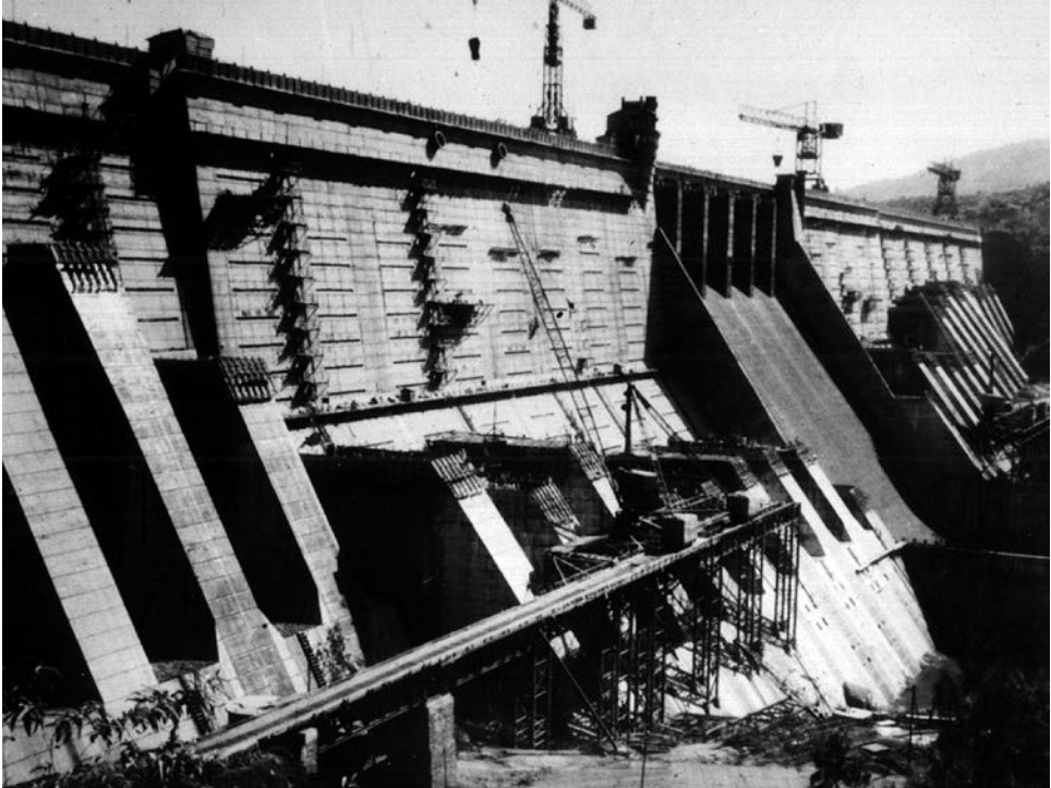
Figure 18.11.4 Addition of buttresses to Koyna Dam after the damage caused by the Koyna earthquake of December 11, 1967. [From A. K. Chopra, "Earthquake Response Analysis of Concrete Dams," in Advanced Dam Engineering for Design, Construction and Rehabilitation (ed. R. B. Jansen), Van Nostrand Reinhold, New York, 1988.]
