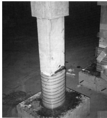
Fig. 2.10 Elliptical jacket filled with expansive mortar at the base of a reinforced concrete column.
