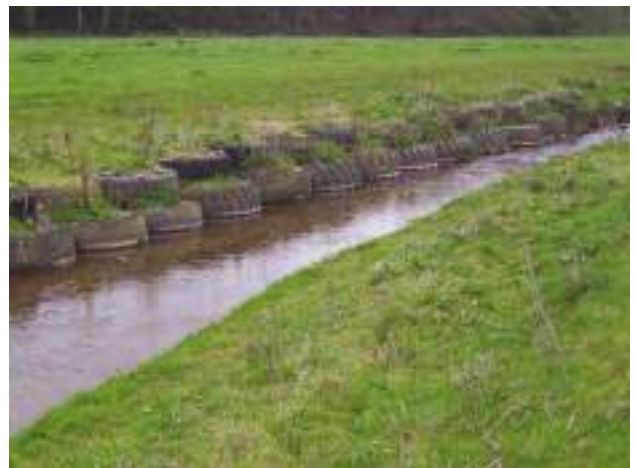
E1Nd Tipped debris – this category includes tyres, old cars, builders waste, and other materials considered as 'waste'. Record also as reinforced (RI).
