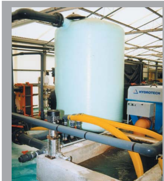
Fig.68.01 Well cleaned biofiltration unit (photo STM Aquatrade)
